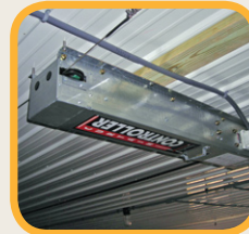
Automated Actuation System
